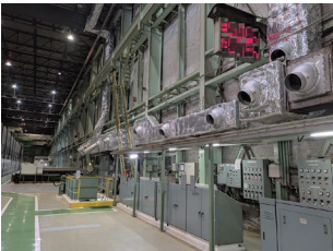
Chiller unit with air supply duct
