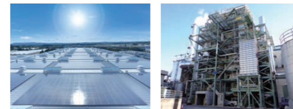
Solar power generation equipment at Rengo's Fukushima-Yabuki Plant | Woodchip biomass power plant at Rengo's Yashio Mill
