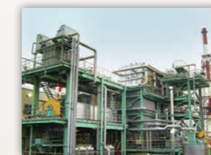
Biomass incineration power plant at Yashio Mill
