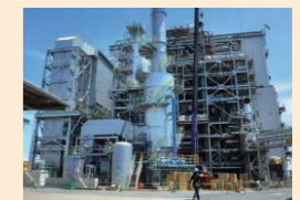
Biomass boiler (within premises of the Tونغewa Division)
