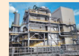
Biomass incineration plant (within premises of the Amagasaki Mill)
