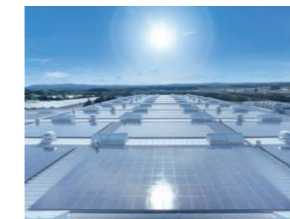
Solar power generation equipment at Rengo's Fukushima-Yabuki Plant
