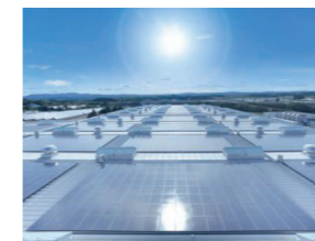
Solar power generation equipment at Rengo's Fukushima-Yabuki Plant
