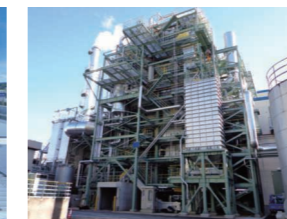
Woodchip biomass power plant at Rengo's Yashio Mill
